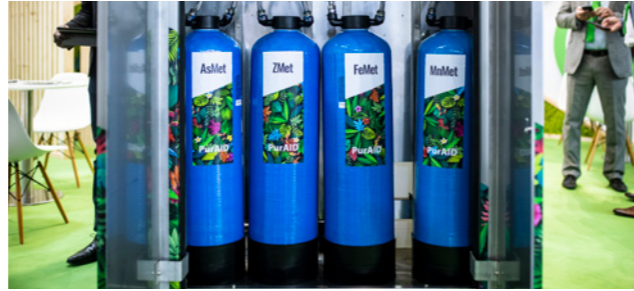
Water purification equipment for container house
